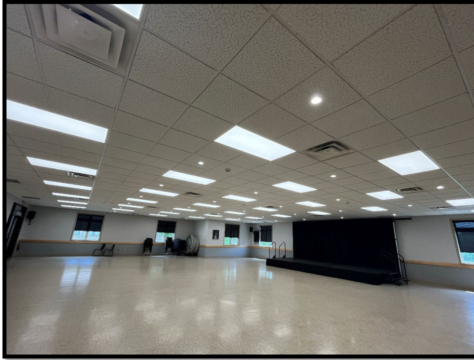
Figure 4: New LED Lighting in Community Hall
